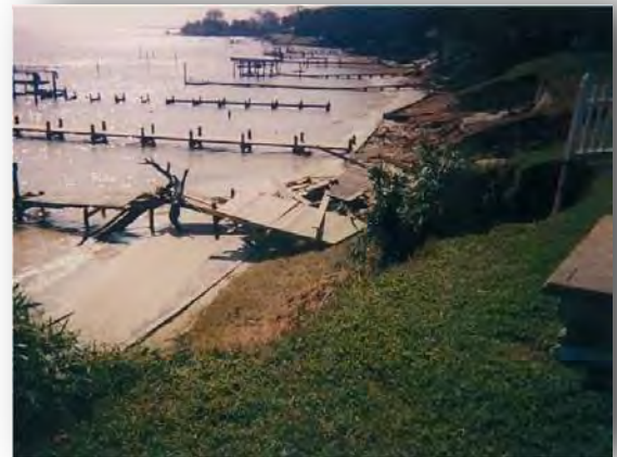
Storm damage incurred on the York River during Hurricane Isabel, 2003. Photo credit: J. Rickards.
